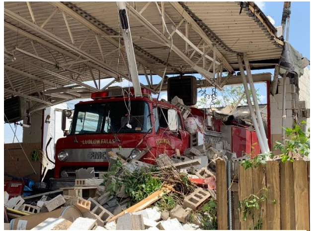
Tornado Damage - J. O'Brien photo
